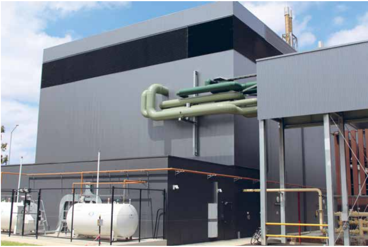
Figure 16-7: Melbourne Airport's Tri-generation Plant – low carbon electricity generation
